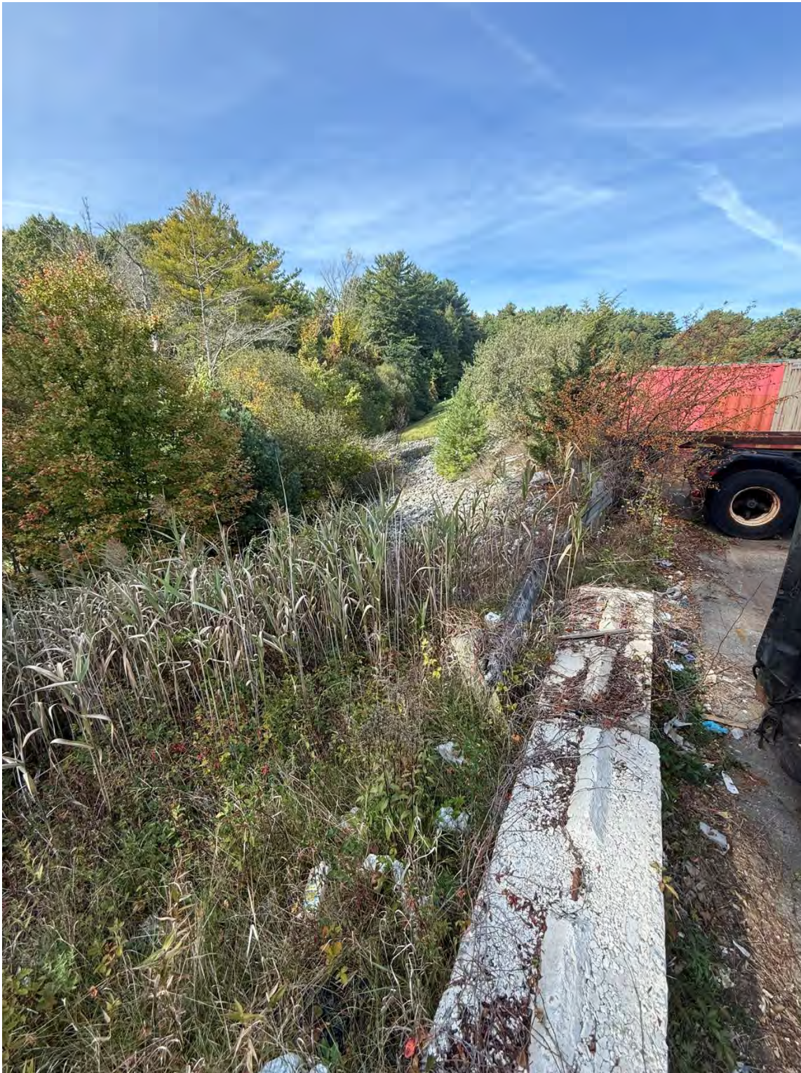
Photo 11: View of the concrete dividers, viewing northwest near the edge of the pavement. Wetland vegetation has grown up the hillside far past the edge of wetlands.
